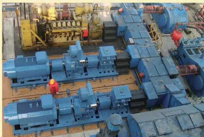
电动机耦合器正车箱动力机组在现场作业 Electric motor coupling gear box power units is operating on site
