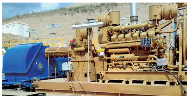
反车箱配济柴柴油机驱动泥浆泵实况 Scenario: Reverse-gear box with Jichai diesel engine to drive mud pump
